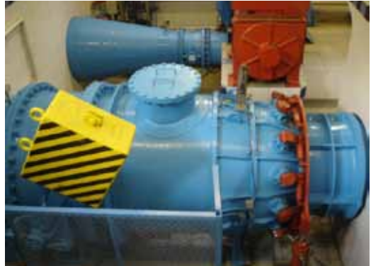
Hydropower installation Prad.
